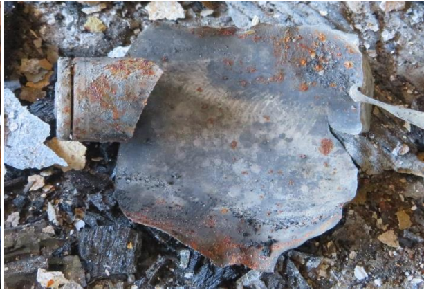
Battery exploded due to thermal runaway
