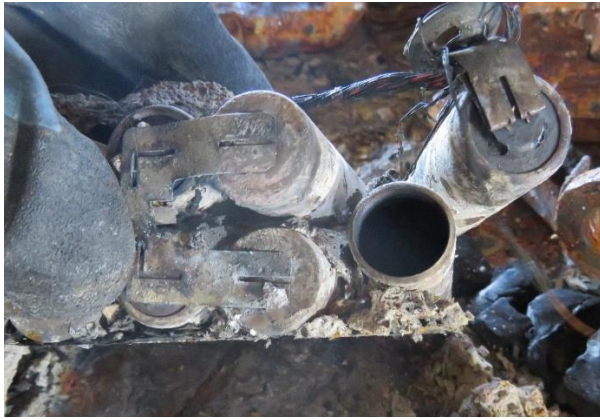
Battery cap blown due to thermal runaway
