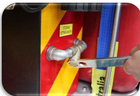
Figure 3.4 - Foam System Strainer
